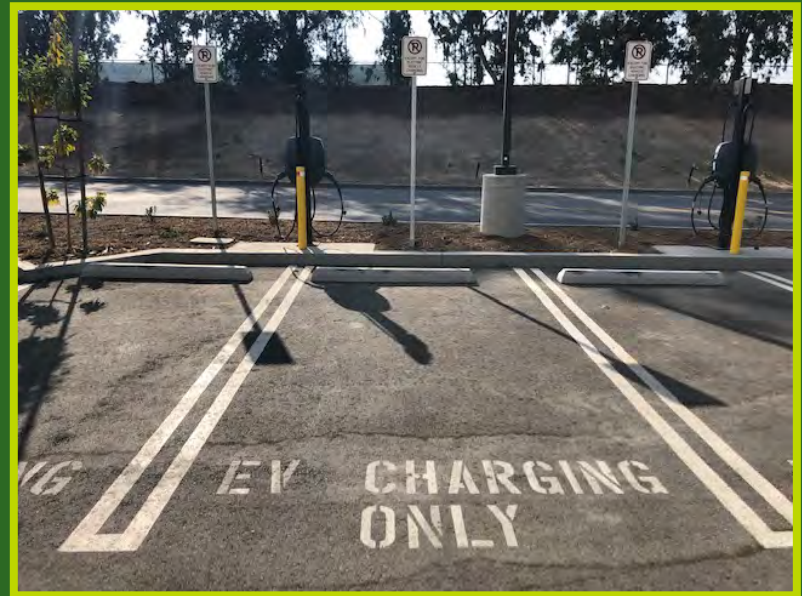
EV Charging Stations
