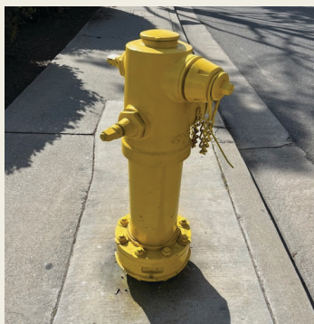
Fire Hydrant with Hydrantguard
