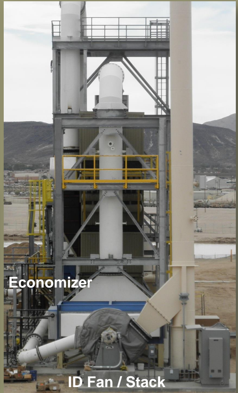
Waste-to-Energy Process Line
