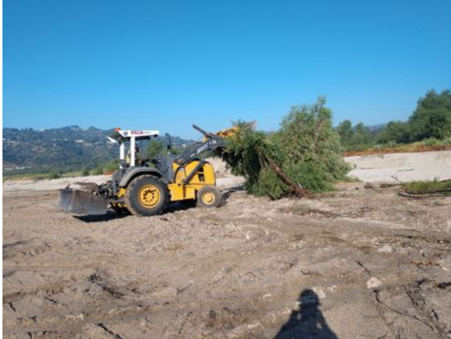
Front-end loader removing vegetation along eastern project boundary near proposed haul road -118.17234 34.19204
