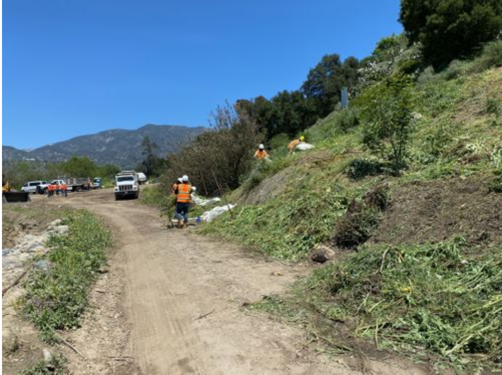
Photo 3_View of road cleared of debris.jpg -118.1732 34.18721
