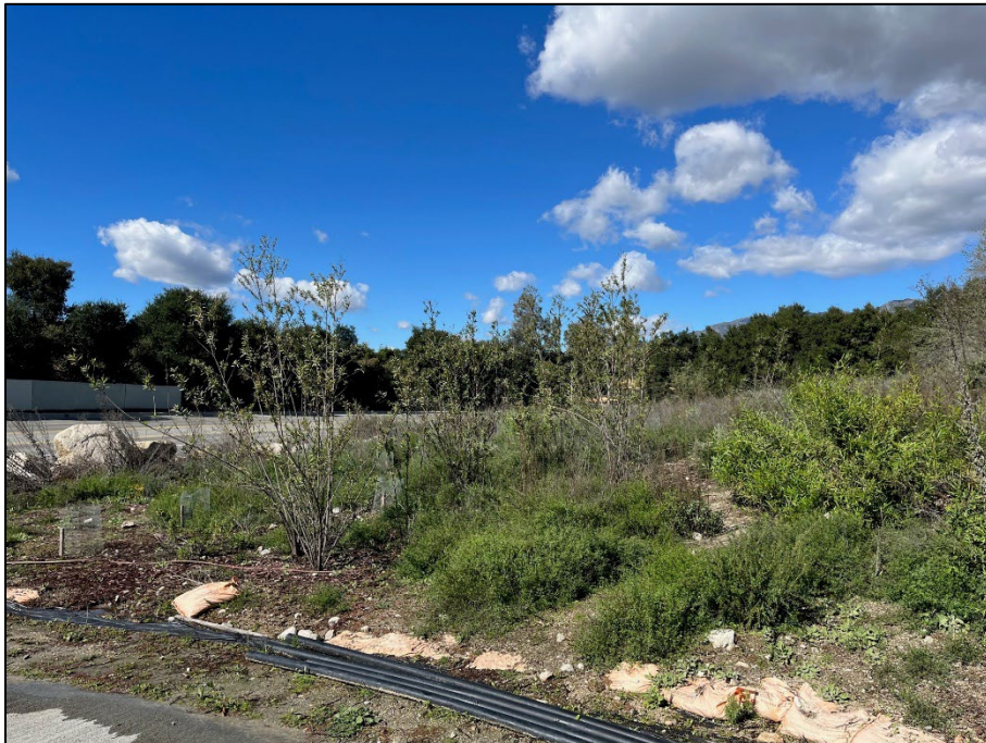
Photo 10: Overview Tire Wash
