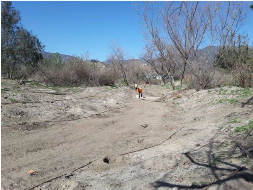
Irrigation set up_DG-2 WOUS_facingN.jpg -118.17235 34.1893
