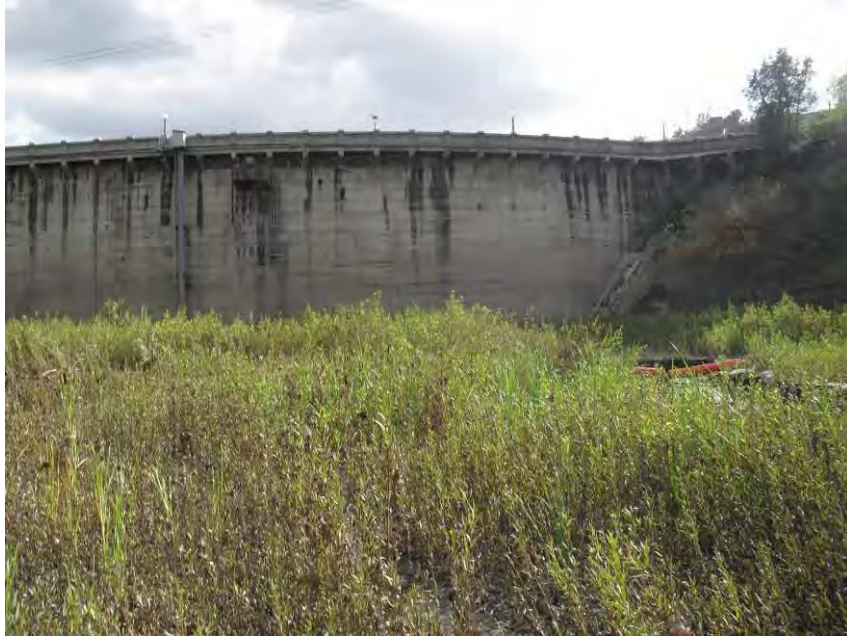
Photo 11: Photo taken from Photo Point 9 looking south depicting the dam wall with emergent riparian vegetation in front of the wall.
