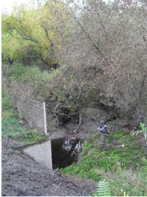
Photo 5: Photo taken from Photo Point 4 looking west depicting a culvert that enters the reservoir on the east side directing neighborhood runoff to the reservoir. A pond existed at the opening of the culvert at the time of the survey with little running water.
